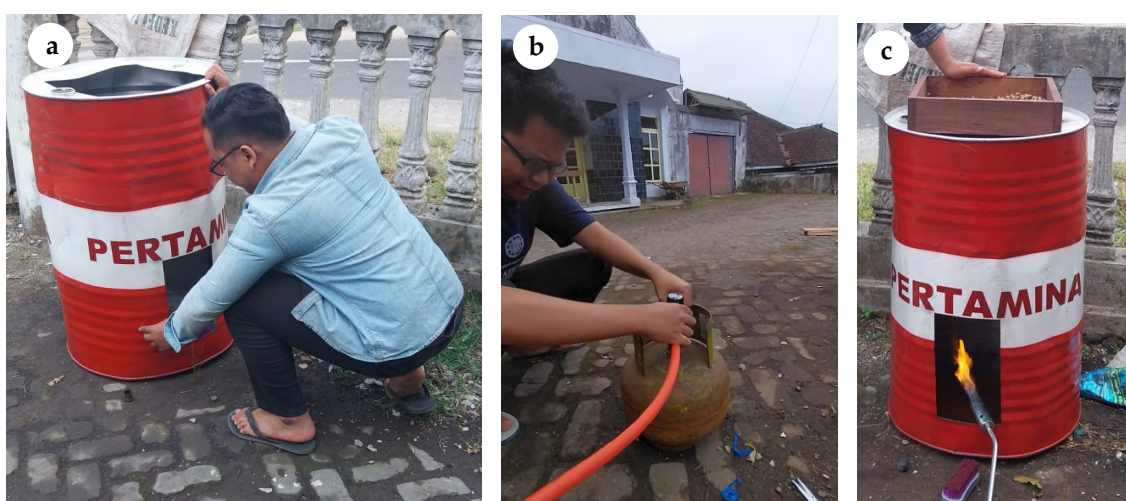
Figure 1. Workshop on creating and operating a javanese cardamom dryer: (a) Cutting and cleaning the combustion; (b) Chamber installing the blow torch and fan; (c) First trial of cardamom dryer
