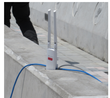
(c) Access point
