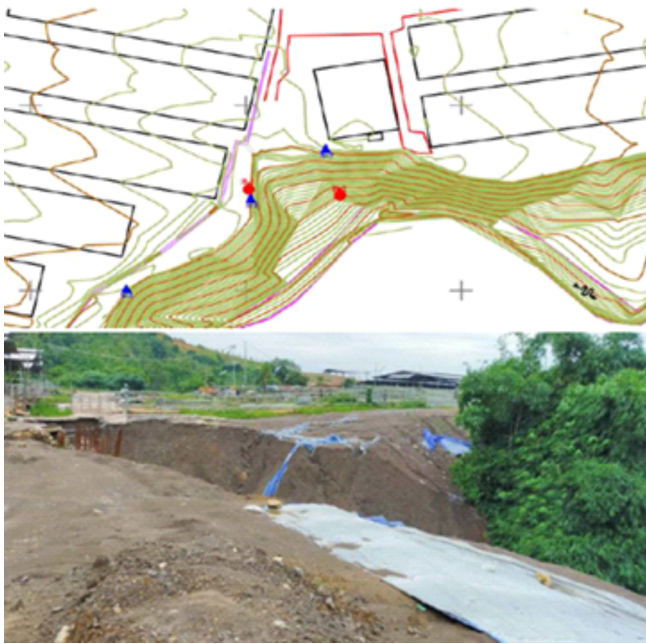
Figure 1 Slope failure on compacted weathered clay shale embankment at Cariu, Jonggol, West Java, Indonesia (Alatas, 2020).
