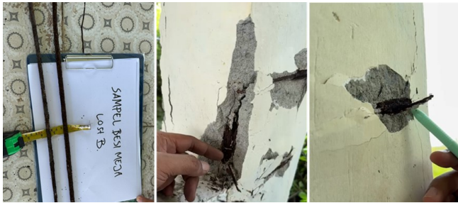
Figure 5 Rebar samples and the condition of corroded rebars that can be fractured
