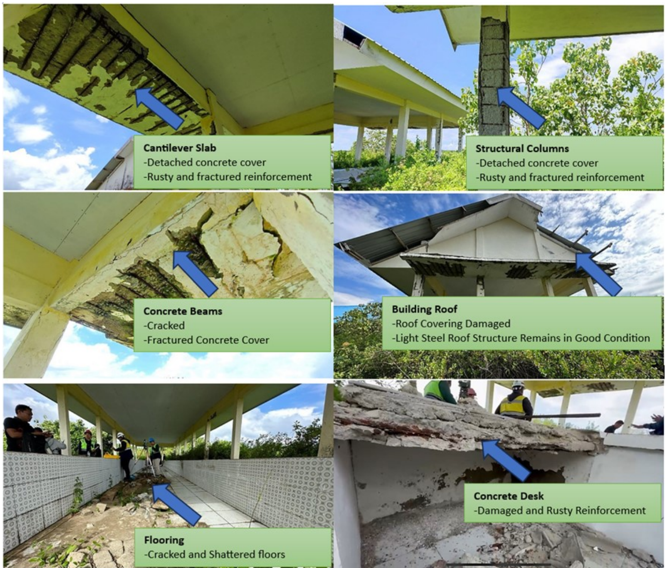
Figure 3 Identification of component damage in the building
