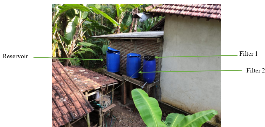
Figure 3. The results of the installation of the filtration system clean water treatment technology.
