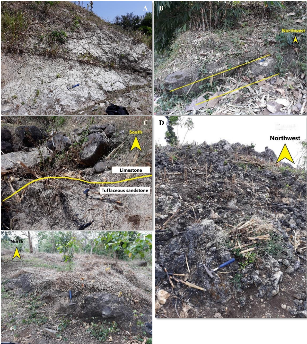
FIGURE 5. (A) The outcrop of tuffaceous marl unit on point station 57. The picture shows a fault cutting the outcrop and a lot of joint (hammer handle points north). (B) The outcrop of tuffaceous calcareous sandstone on point station 1. The outcrop shows the bedding plane N179°E/28°. (C) The outcrop of contact lithology between limestone and tuffaceous sandstone at point station 29. (D) The outcrop of grainstone-mudstone unit at point station 48. (E) The outcrop of andesitic breccia at point station 41.
