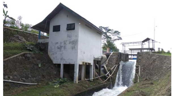
Figure 1. The condition of PLTMH Blumbang
